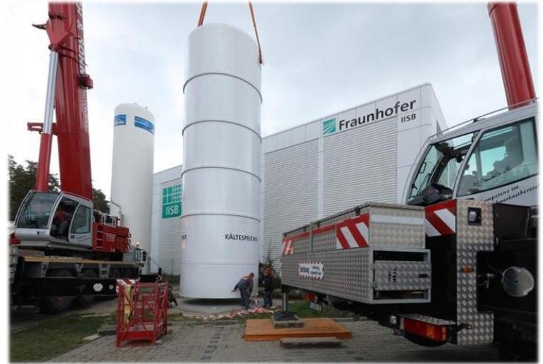
80 m 3 vacuum isolated cold energy storage at Fraunhofer IISB
